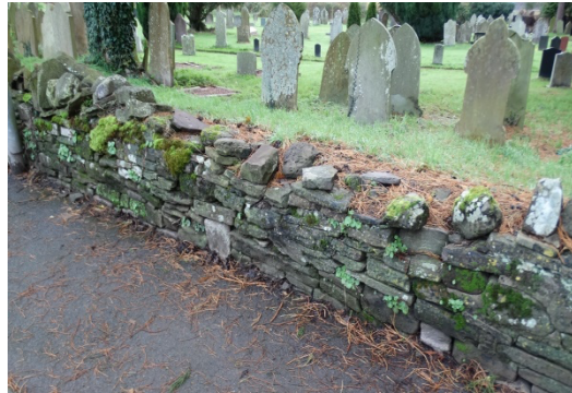
Broken walls & boundary fences
